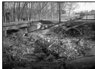
Bridge debris from trash
